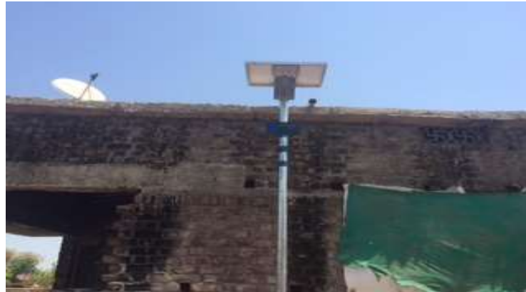
Solar Panel installed -
